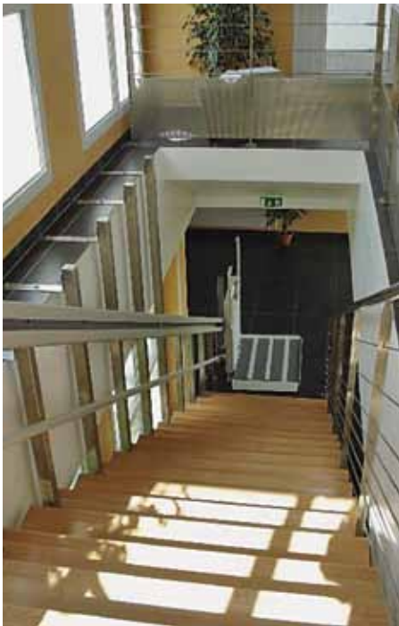
Indoor installation, top level mounted stanchions. France.
