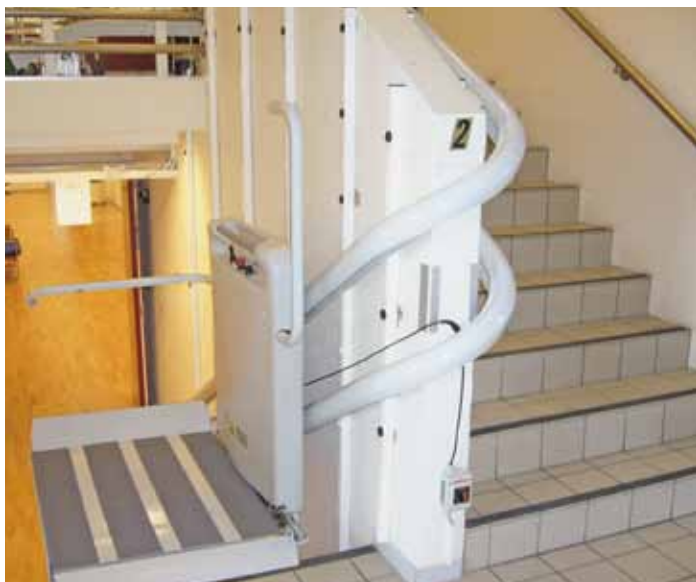
Indoor installation 180° bend on landing. Public building, Denmark.
