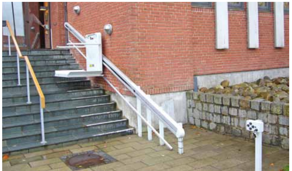
Outdoor installation: partly wall, partly stanchions. Call station on separate stanchion. Church, Denmark.
