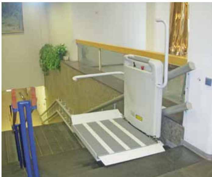
Indoor installation bend over horizontal landing. Factory in Finland.
