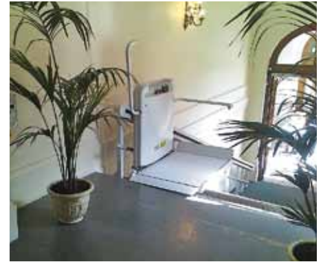
Indoor installation on stanchions. Public building, France.
